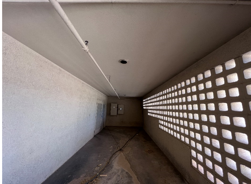
EXISTING UTILITY METER AND FUSED DISCONNECT
